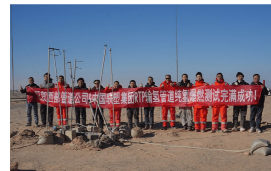
輸氫管道純氫爆燃測試圓滿成功 Successful Completion of Pure Hydrogen Deflagration Test of Hydrogen-transporting Pipes
