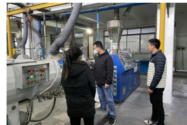
改進供應商排水管析出問題 Improvements to Crystal Precipitation in Drain Pipe for Suppliers
