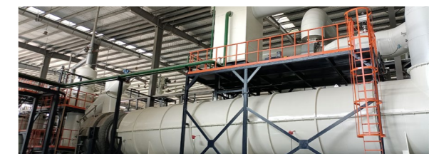
污泥熱解系統 - 連續爐 Sludge Pyrolysis System - Continuous Oven
